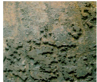
Under Deposit Corrosion
