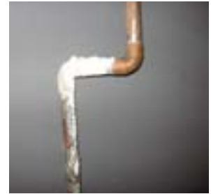
Hard scale build up on exterior of copper pipe in plumbing system.
