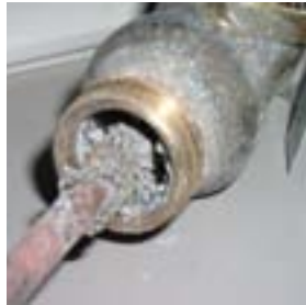
This temperature and pressure relief valve has become clogged with the accumulation of hard scale, which can lead to potentially dangerous conditions.
