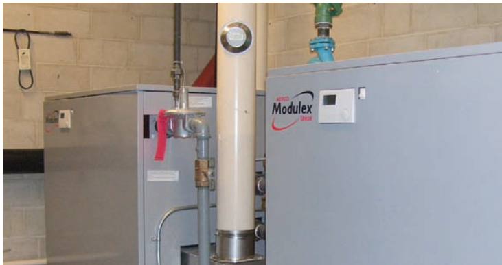
Replacing Graystone Corporation's existing atmospheric boilers with AERCO condensing boilers significantly reduced boiler room operating costs.
