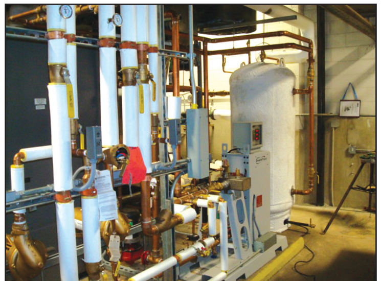
The new system with a SP33 heater and 200-gallon boiler-side buffer tank.
