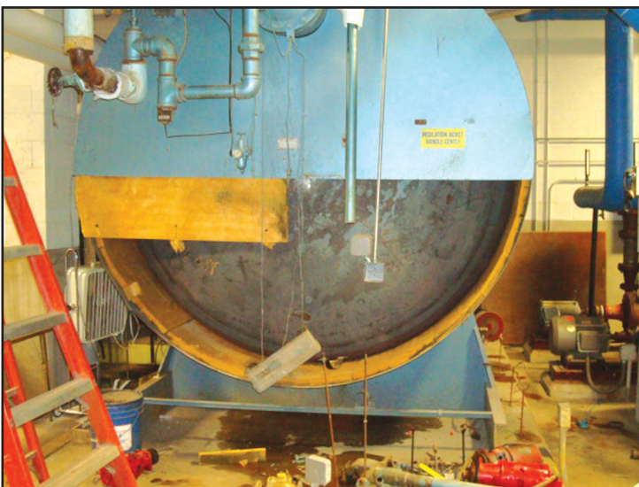
The previous system required a 5,000-gallon storage tank, shown above.
